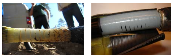
a) Incorrect peeling of the isolation with visible PD-tracking, joint close before failure b) Remaining semi-conductive layers
